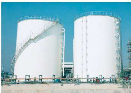
Long liquid tank
